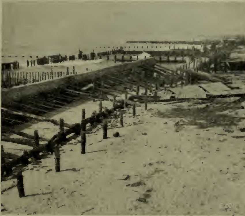
FIG. 2. SHOWING SCOUR BEHIND VERTICAL PILING.
